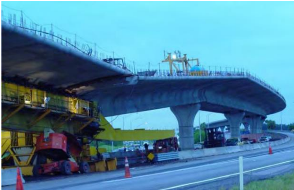
Figure A-10: Collapse of Pier 97 in April, 2004 (Graham et al., 2014)
