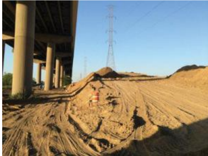
Figure A-6: Tilting bridge piers and adjacent soil stockpile (O'Shea, 2015)
