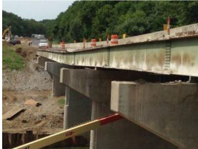
Figure A-8: Post-Failure View, I-65 Bridge, Lafayette, Indiana (McCoy, 2015)
