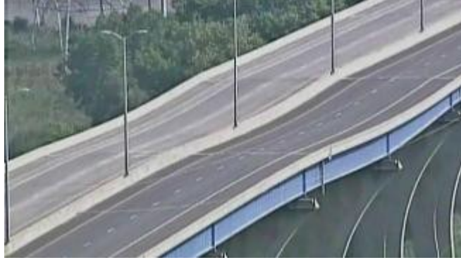
Figure A-2: Sagging Leo Frigo Memorial Bridge (Thompson, 2013)
