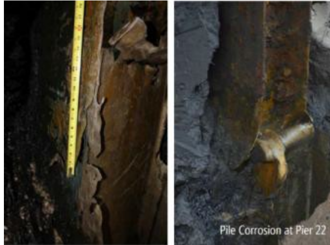
Figure A-3: Pile Corrosion at Pier 22 (Source: Wisconsin DOT)
