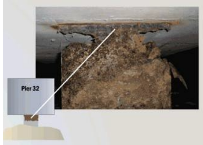
Figure A-14: Pile corrosion under Pier 32 (Paint Square, 2013)
