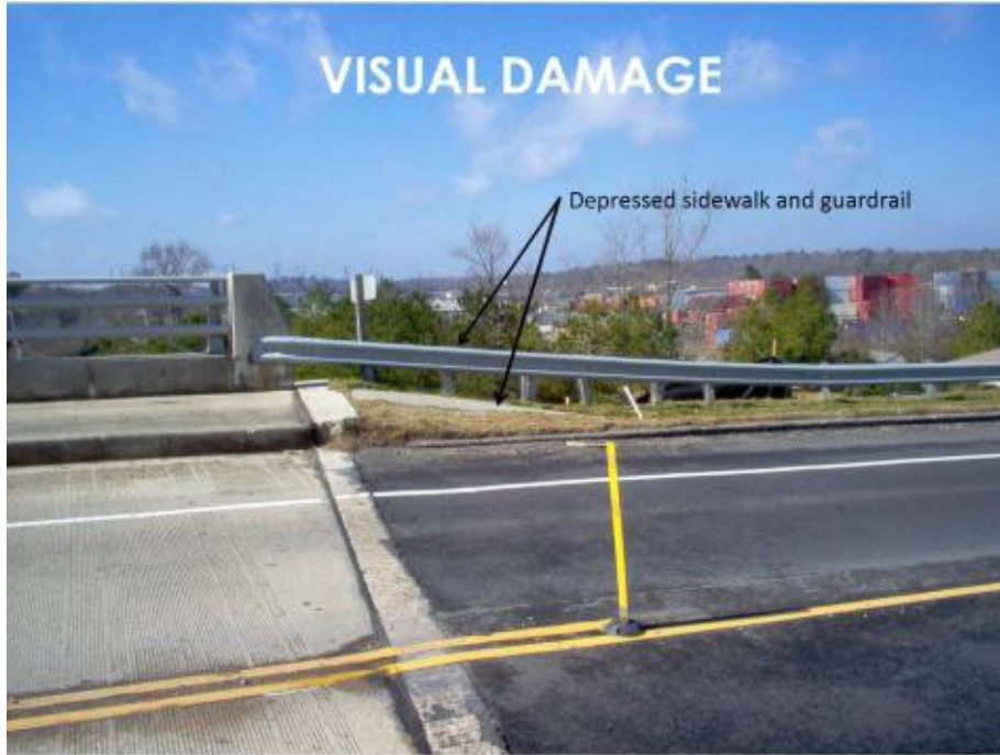
Figure A-16: Damage from Settlements (DeStephen, 2015)
